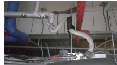
Case of draft failure
